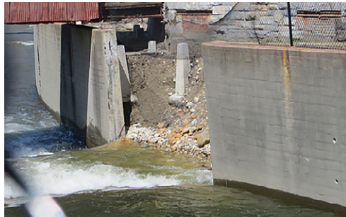
Flood Control status: the latest concrete panels to fall is adjacent to MASS MoCA Bldg 6
